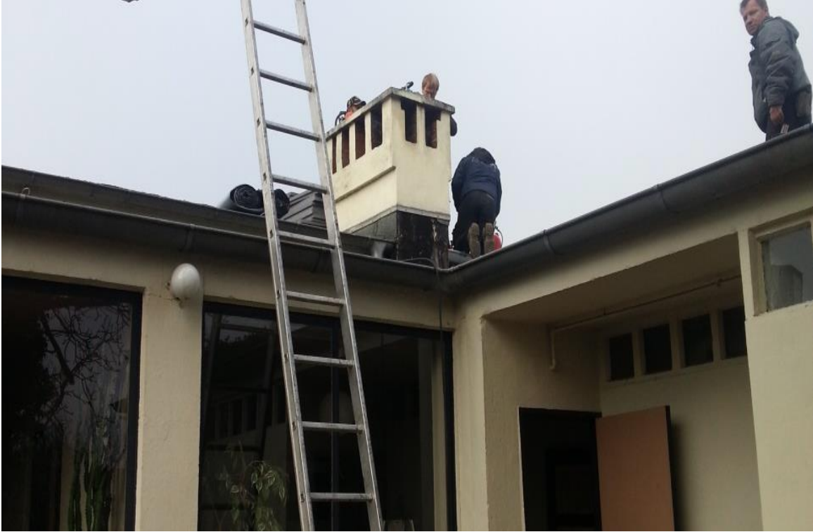
Figure 9: Contemporary installation in progress, which is against the conservation rules.
