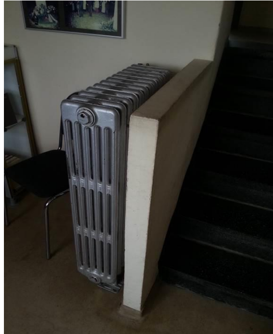
Figure 12: The additional heating insulation at semi-basement service area, 43 Mittlering. (Middle ring) Source: Sayed Ahmed during survey in 2016
